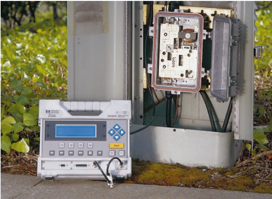
HP CaLan's Sweep/Ingress Analyzer at work in the field
