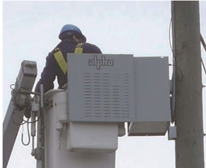
Figure 2 – Typical Utility Pole Mounted Broadband UPS
